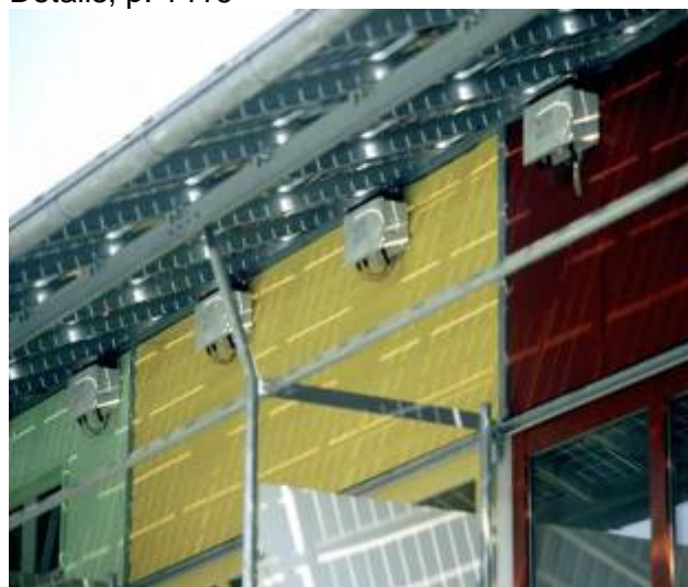
Row of inverters (copyright ©2007: Ingo B. Hagemann)
