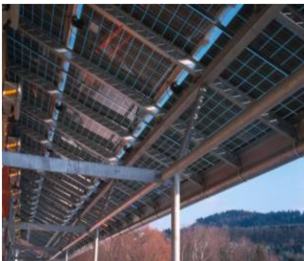
Underneath view of support structure for PV-Modules (copyright ©2007: Solarsiedlungs GmbH)
