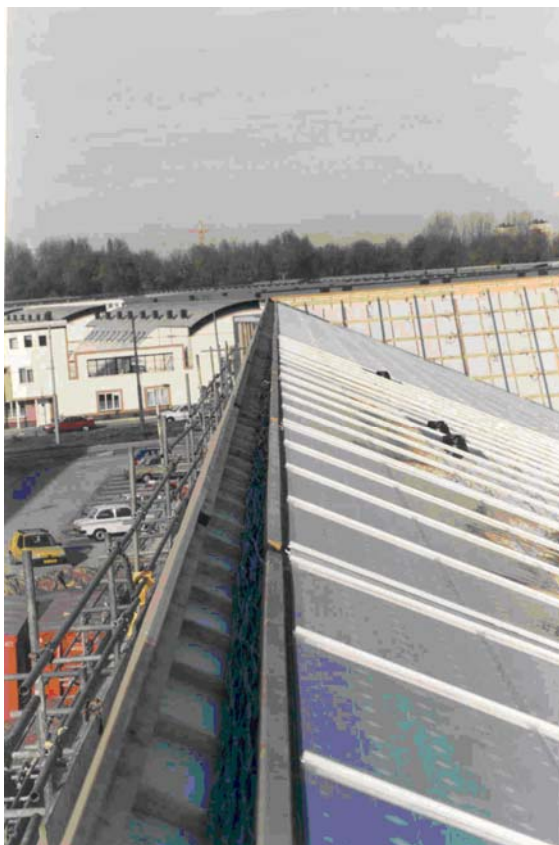
Photo 4: The string cables are collected in the cable duct along the ridge side of the roof.
